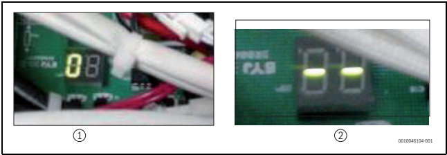
Fig. 22 Main board LED when power on and in standby
